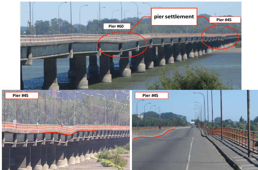
Figure 2-5 Juan Pablo II Bridge: Observed pier settlements (from Ledezma et al., 2012).
