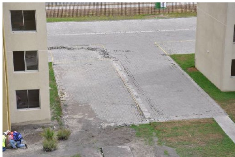
Figure 2-14 Ground settlement between the Riesco and Bulnes Buildings (from Bray & Frost, 2010).
