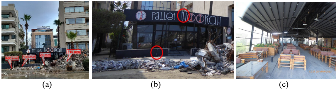
Figure 2-23 (a) Buildings K, L and M in Area 2 with Building L in the middle; (b) damage to the exterior at Building L due to the hogging deformation; (c) damage to the concrete slab at Building L due to the hogging deformation (from Moug et al., 2024).
