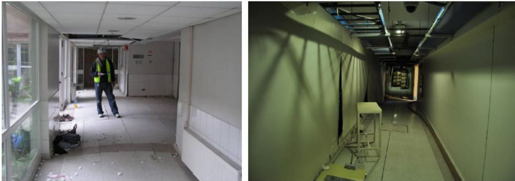
Figure 2-11 Floor distortions and bulging observed at Curanilahue Hospital (from Bray & Frost, 2010).
