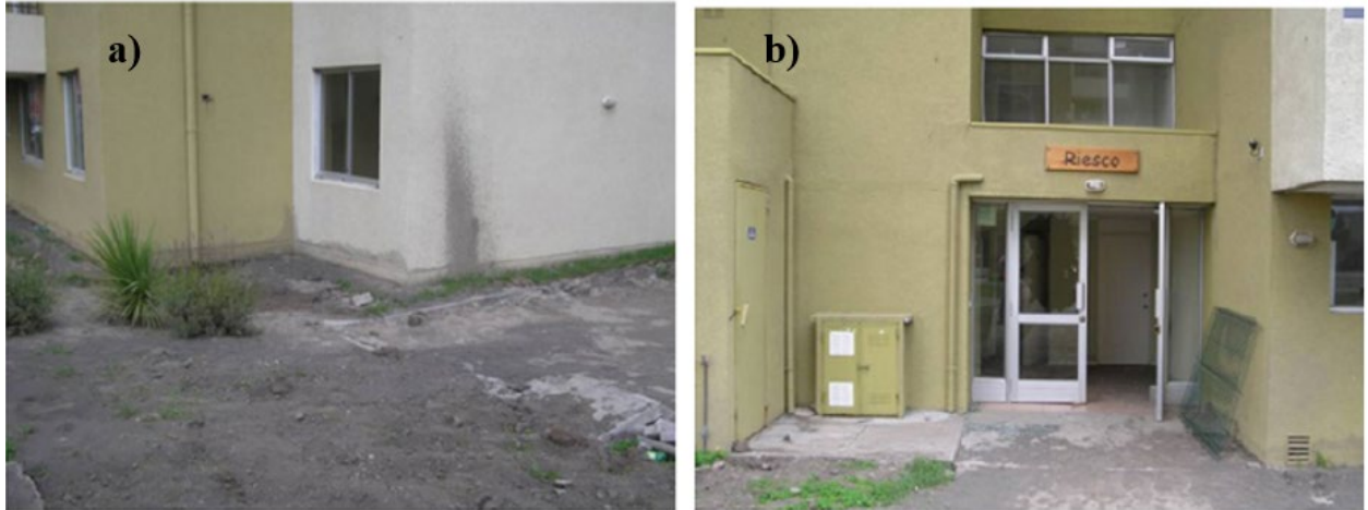
Figure 2-13 (a) Evidence of large sediment ejecta at the northeast corner of the Riesco Building; (b) Entrance to the building in the middle of its east facing side with 1° tilt observed in the coupling beam (from Bray & Frost, 2010).
