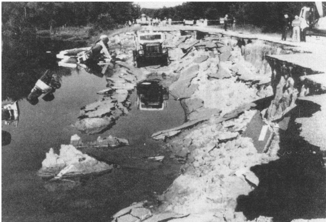
Figure A.9.2: Photograph showing the failed embankment (looking towards the west), showing crest loss and the positions of four of the large geophysical exploration trucks. (Hryciw et al., 1990).
